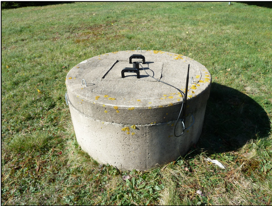
Figure 8: External antenna mounted on side of well with cable leading to meter inside well.
