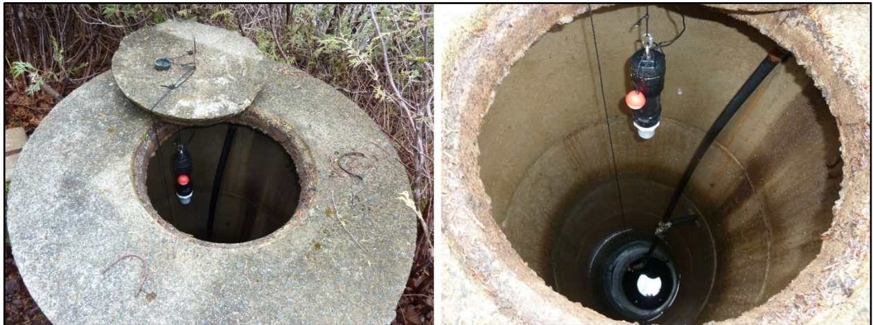
Figure 10: Meter installed in a dug well.
